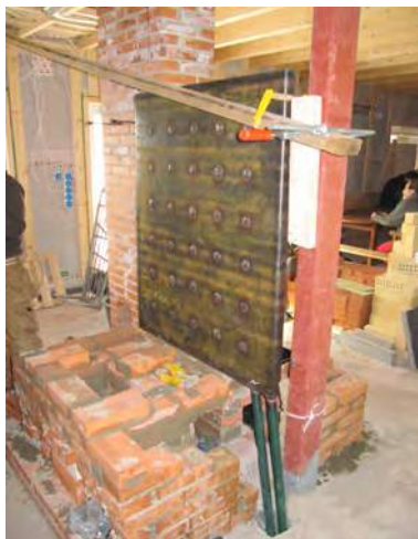
Masoning the heat storage fireplace. The water heater component located in the middle. Photo by Ella Suhonen.
