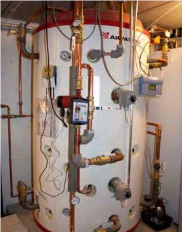
The water accumulator located in the cellar, underneath the fireplace. Photo by Ella Suhonen.
