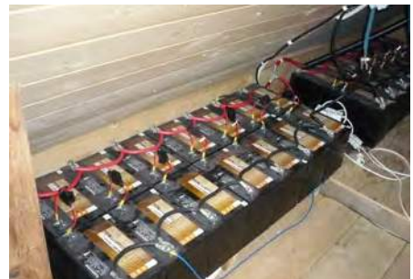
Electricity storage system (12V battery bank). Photo by Karl Gunnar Randau.
