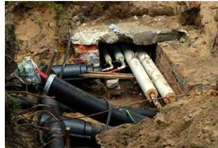
New well-insulated pipes (black) replace the old system (white). Photo by Achim Ecker.
