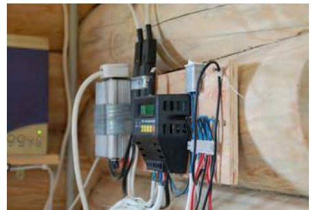
Electricity distribution system in family house. Photo by Daina Saktiņa.
