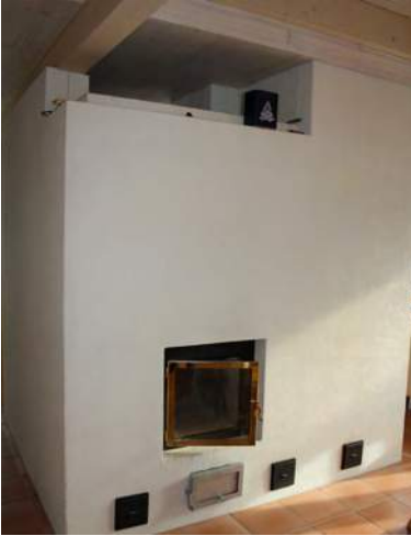
The heat storage fireplace construction and the low-emission firebox. Photo by Ella Suhonen.
